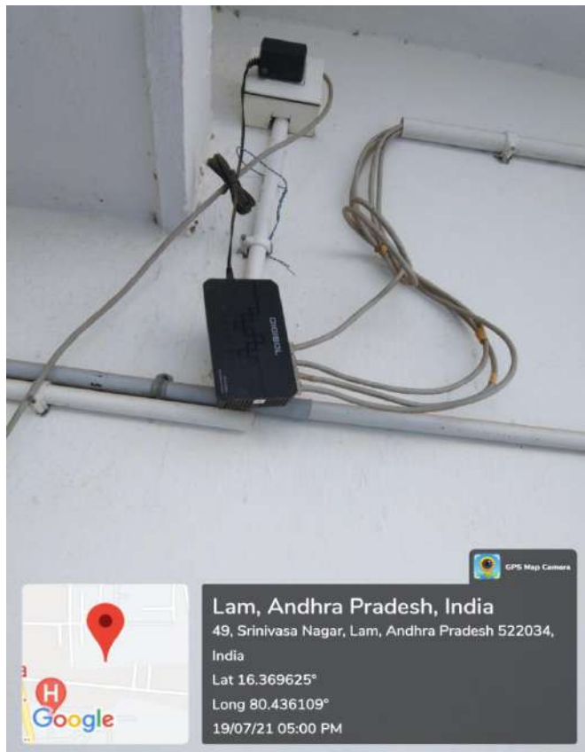
Router-First Floor in Seminar Hall Block
