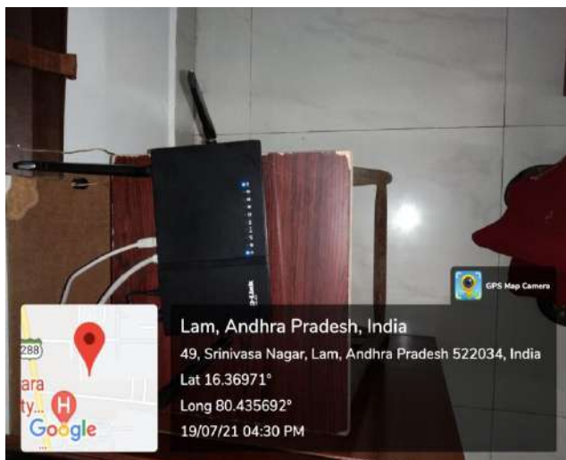
Room No: 112 Boardroom Router
